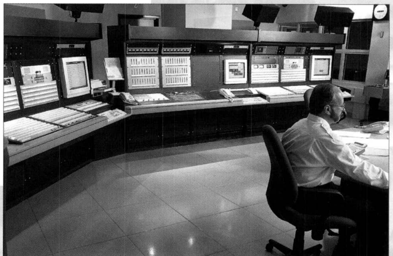
Radio master control, Canadian Broadcasting Centre, Toronto.
